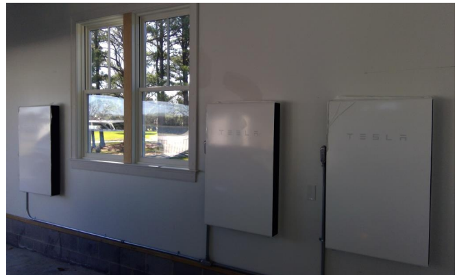
Figure 4 Tesla PowerWalls in garage
