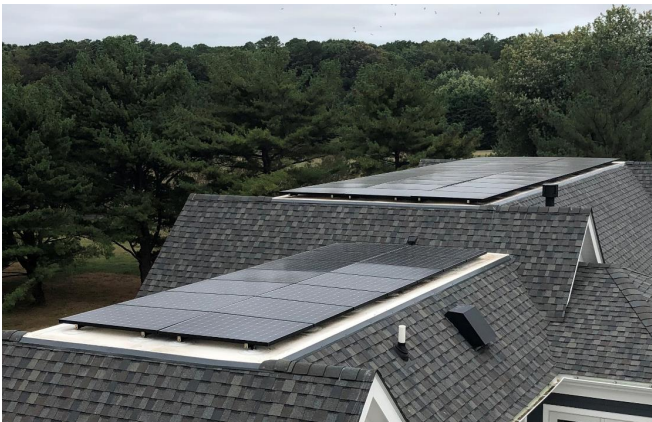
Figure 3 Solar PV array atop the house
