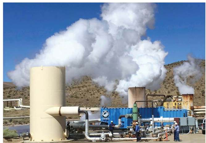
Figure 2. GreenFire Energy’s demonstration of a Closed-Loop Geothermal (CLG) energy system at the Coso, California geothermal power plant. September 2019.
